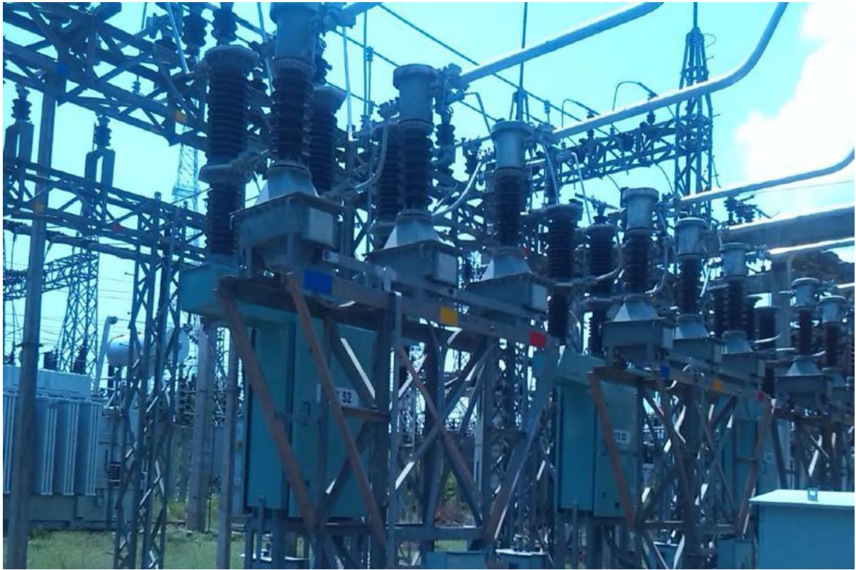
A View of the Renovation and Modernisation works carried out at Villianur 110/22KV Sub-station at Puducherry.
