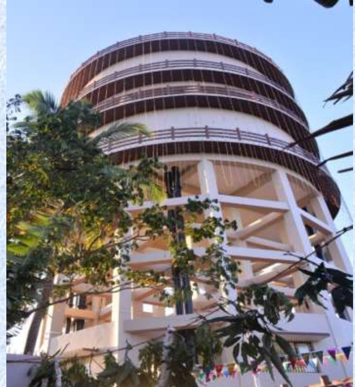
Double Decker Circular OHT with a capacity of 10 lakh litre was constructed at Ariyankuppam.
